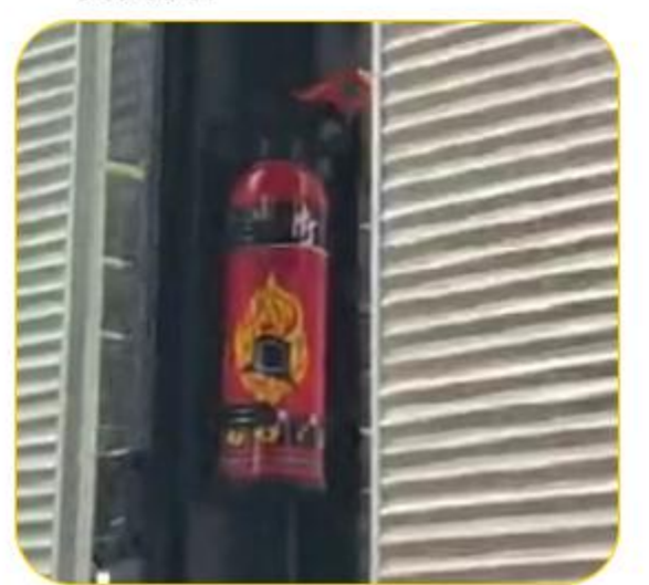
Equipped with fire extinguishers.
